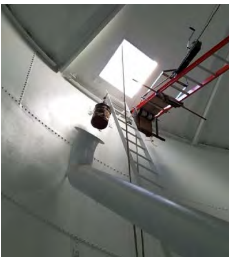
Water tower 2 received a fresh coat of interior paint as part of the improvement project.
