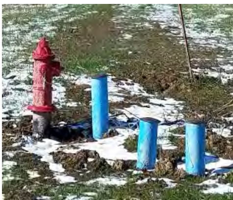
New fire hydrants and isolation valves were installed by Branco Enterprises, Inc.
