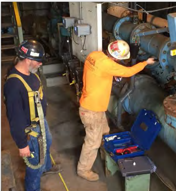
MCA Construction crew members prepare to replace 18 valves at the water treatment plant earlier this year.
